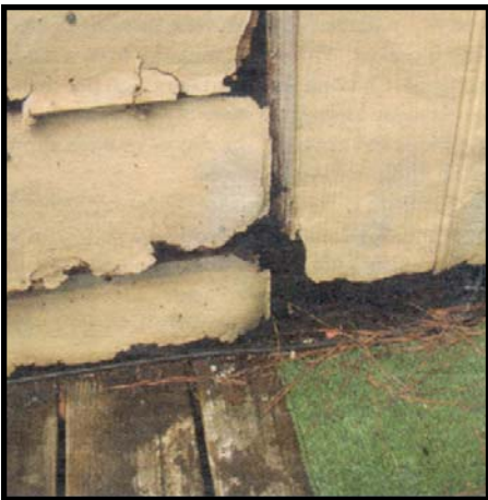
Building damage from Hurricane Floyd flooding. Photo by York Wilson, The Independent Weekly , reprinted with permission from a Sept. 4, 2004 article: www.indyweek.com/gyrobase/Content?oid=oid%3A22560 .
